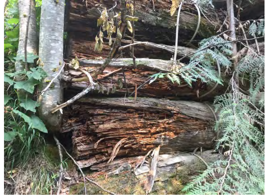
Log crib condition
