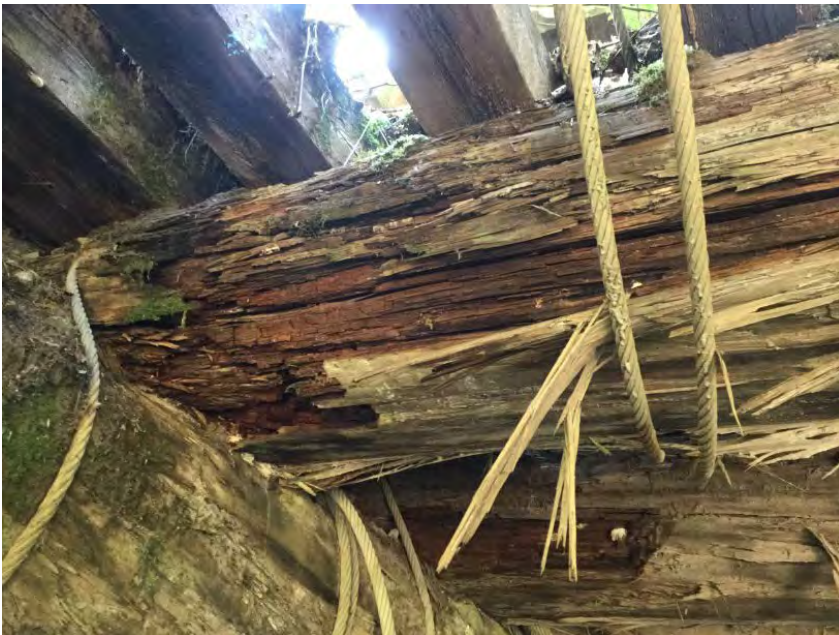
Log stringer condition
