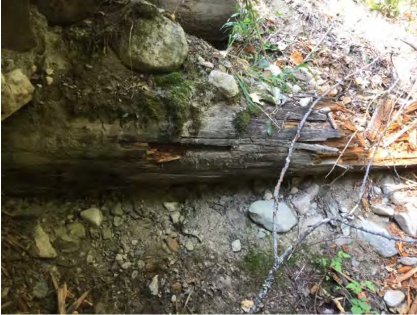
Upstream right bank sill condition
